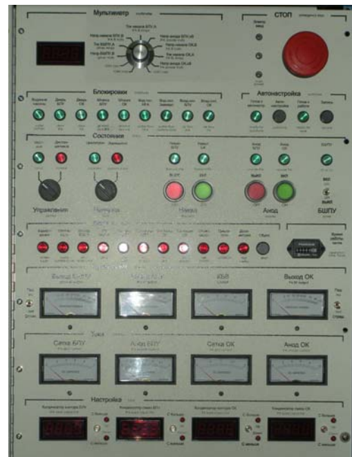
20 KW, 6.5-12.5 MHz, RF Amplifier for JINR Front Panel
